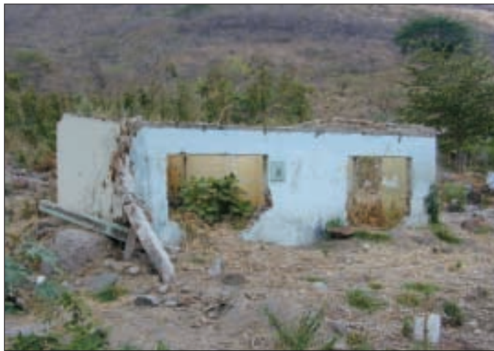
Figure 5. Structures destroyed by debris flows behind hospital at La Trinidad.
