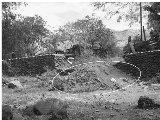
Fig. 5 Image of a filling on La Trinidad river bed indicated with a white circle. The dike, built after the Mitch hurricane event, presents a discontinuity and erosion is beginning to act behind it (white arrow). The lower terrace level is indicated with a white discontinuous line. La Trinidad, 2004
