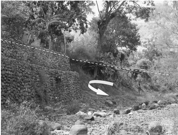
Fig. 4 Image of the concave margin of a meander. Undermining is evident below the roots of the tree, where unconsolidated sediment is being eroded (white arrow). The dike, built after the Mitch hurricane event, is obviously too short and undermining is beginning to act behind it and therefore it will be ripped off. The lower terrace level is indicated with a white discontinuous line. La Trinidad, 2004
